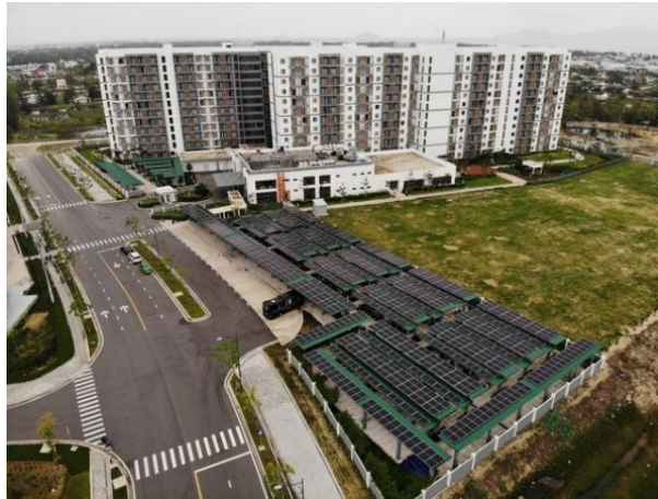
Picture 5. A part of the solar panel system in Hoiana
